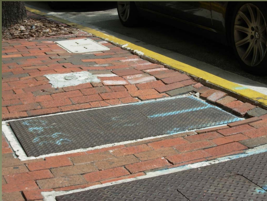
Lifting & settlement of clay pavers
