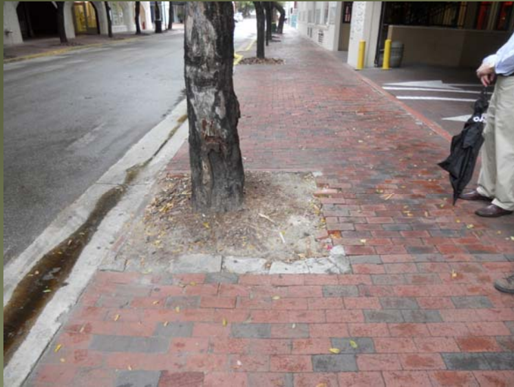
Undefined and uneven edges
