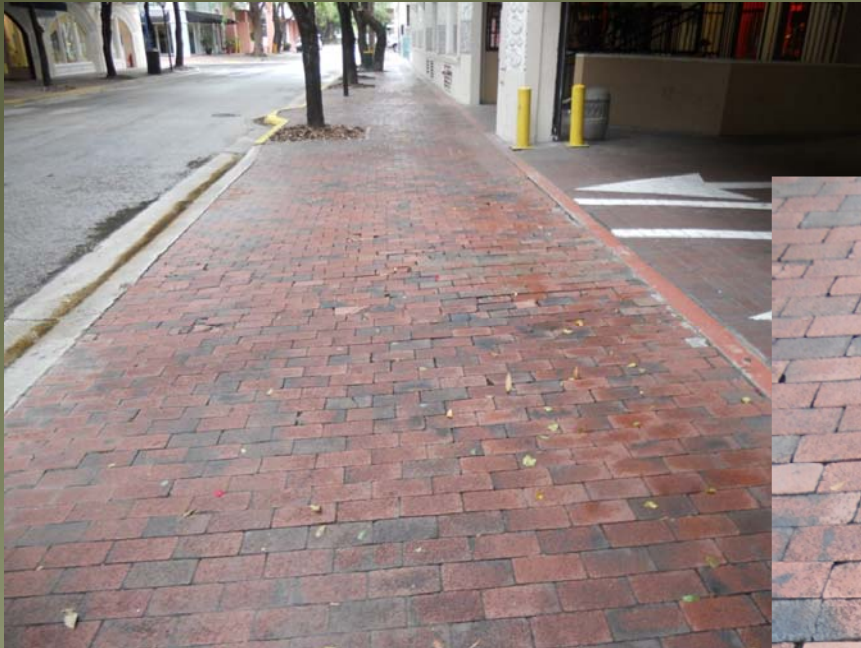
Broken clay pavers at driveways
